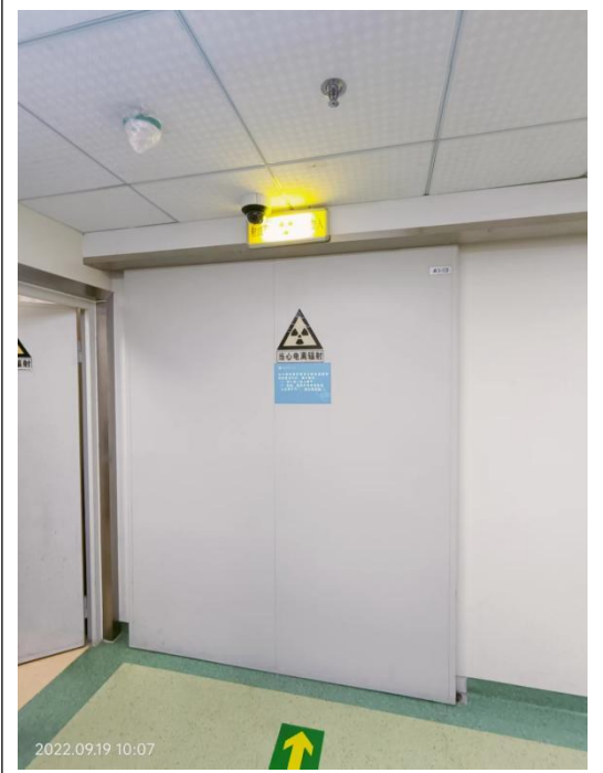
PET/CT 机房警示灯
